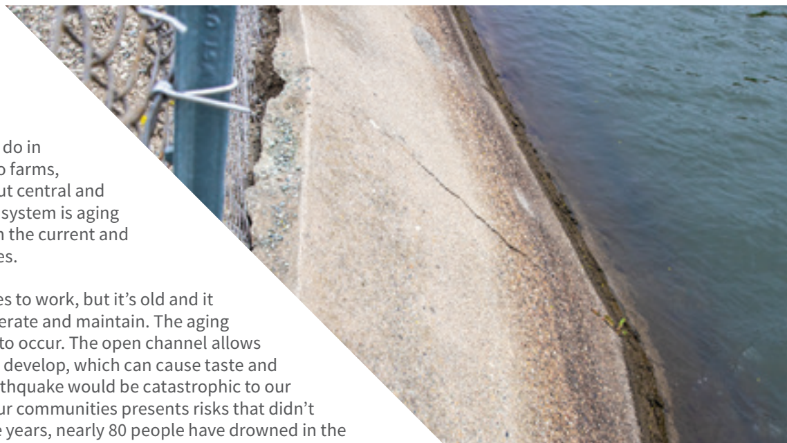
Cracks and buckling panels along the canal's liner reveal its age.
